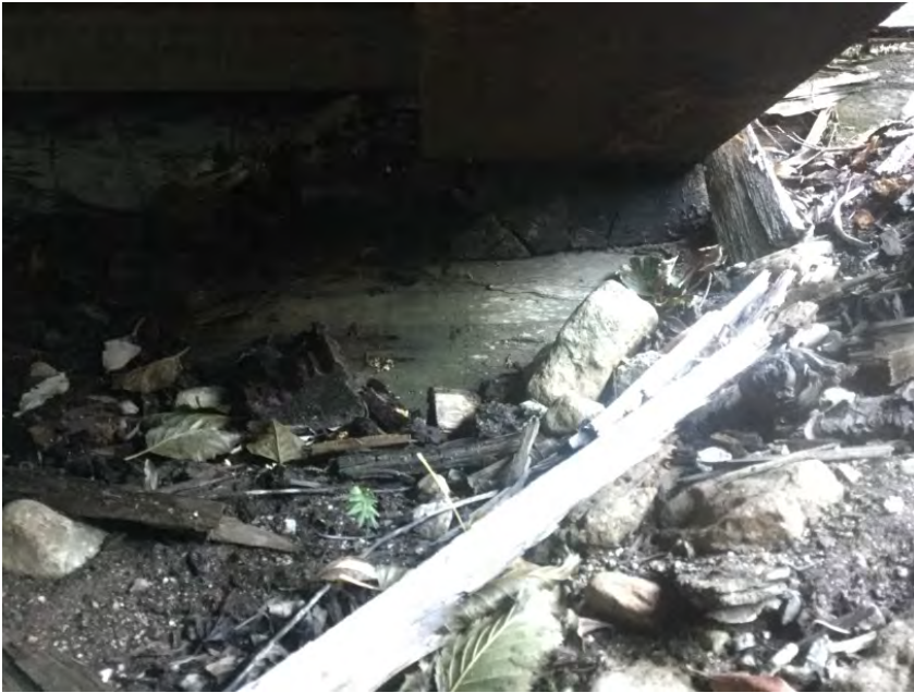
Left bank timber shims rotten
